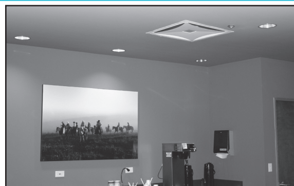
Spectrum diffuser installed in the ceiling of a conference room
