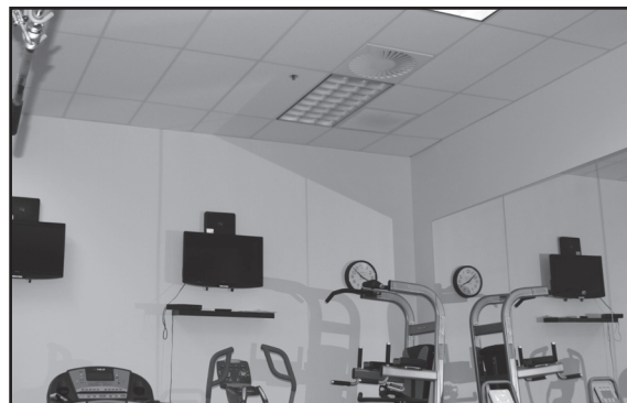
TSW installed in ceiling of a workout facility
