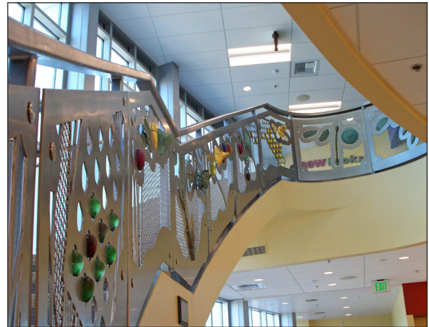
MCD diffuser installed in the ceiling of a library
