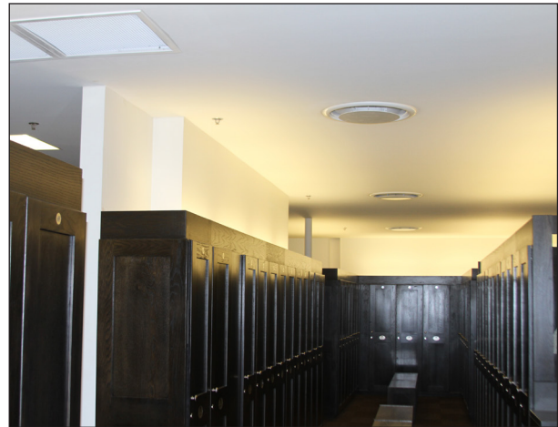
Several R-OMNI diffusers installed in a locker room
