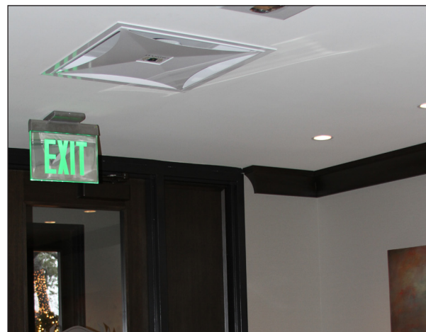
Spectrum diffuser with logo inset installed in an upscale country club
